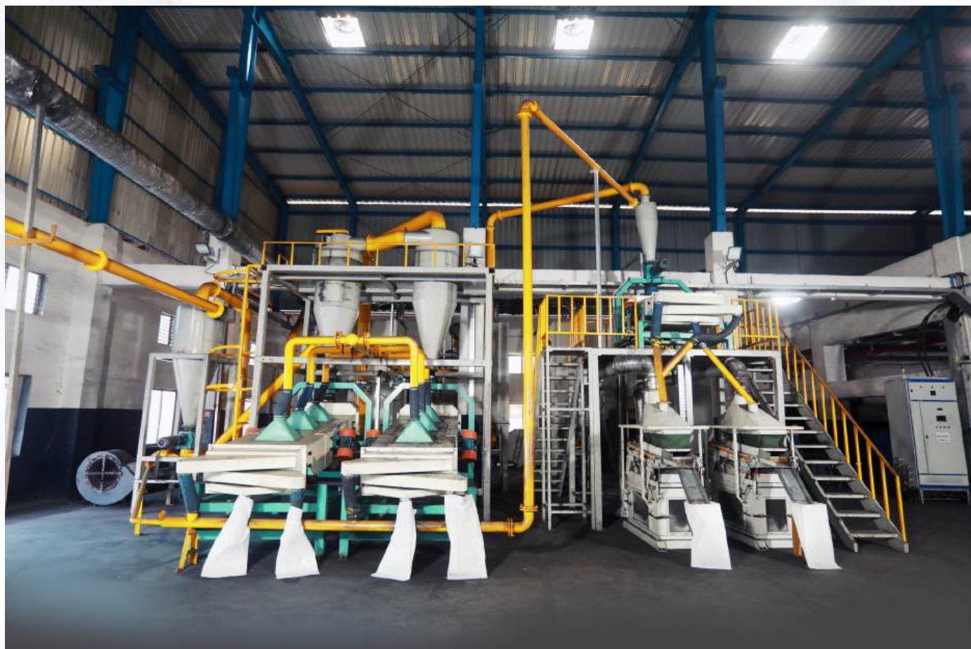
Image: Lico Materials recycling plant in Mumbai
